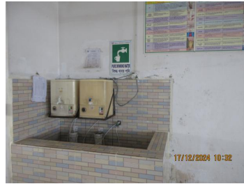
Drinking water area.JPG
