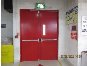
Fire Exit Door.JPG
