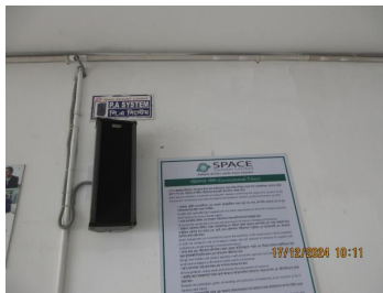
Public Addressable system.JPG
