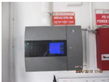
Fire control panel.JPG
